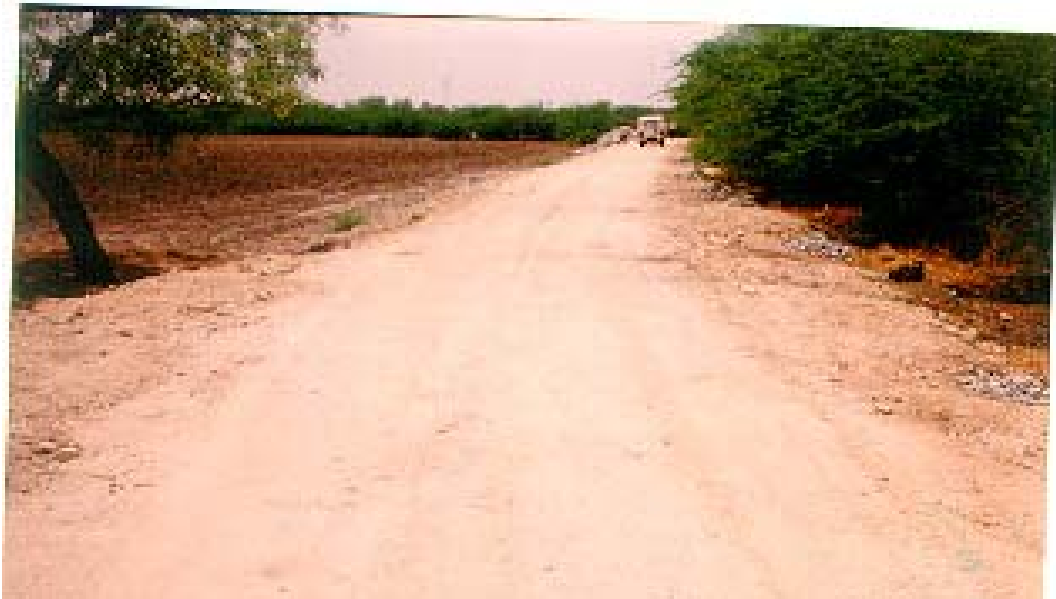
Two Km stretch of Raichur- Arsnagi road, via Yadlapur in Raichur distt. of Karnataka. The fly ash road (in unmetaled condition) has performed well for last 3 years.
