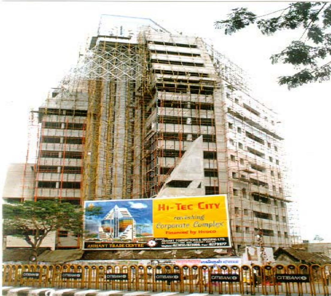
Use of flyash based cellular light weight concrete at Hyderabad, Andhra Pradesh
