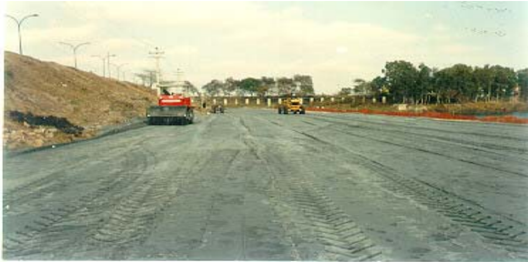
Nizamuddin bridge approach road embankment at New Delhi (in flood zone of river Yamuna)
