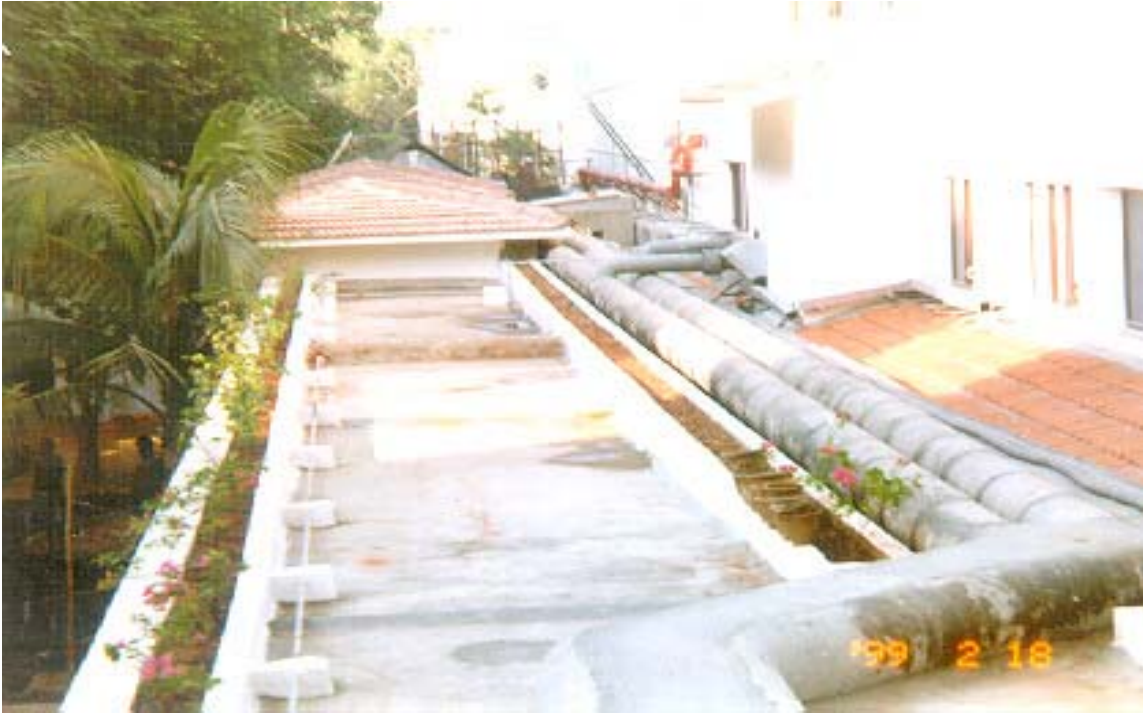
Use of fly ash based cellular concrete in at Chennai, Tamil Nadu
