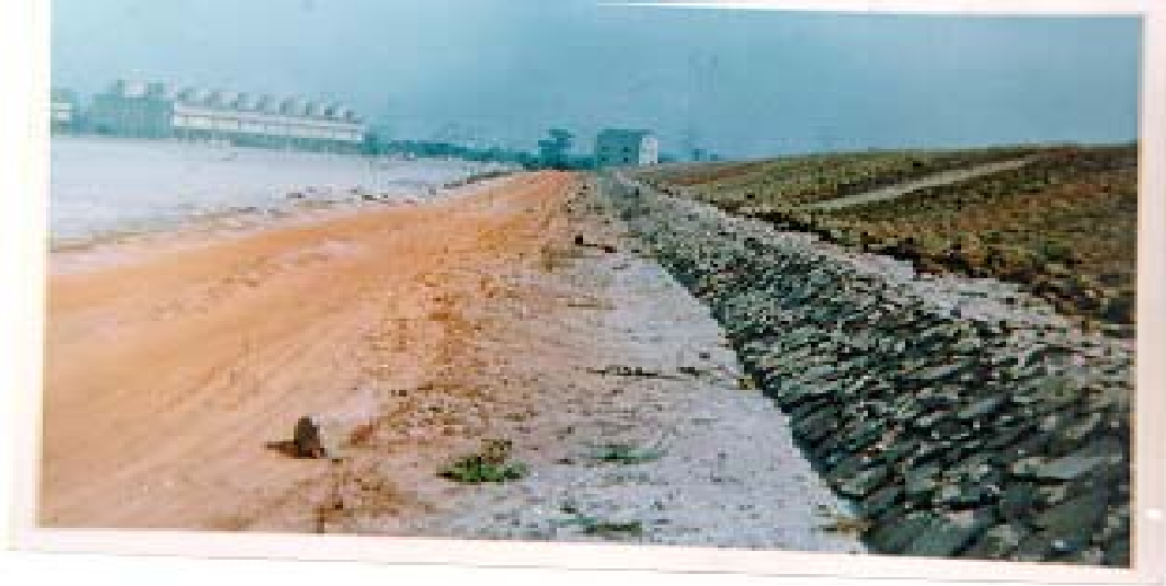
Dyke constructed with fly ash at Korba Thermal Power Station, Madhya Pradesh
